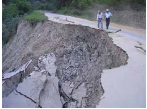
Collapse of Road Caused by Rain Water Bermejo, SCZ on Route 7 (February 2007)
