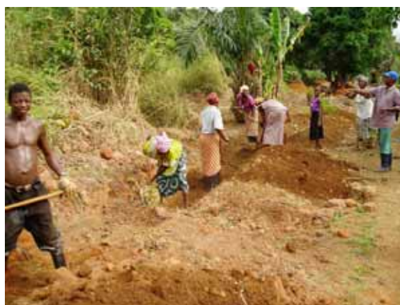
Excavation carried out by the Participation and Collaboration of the members of Pilot
