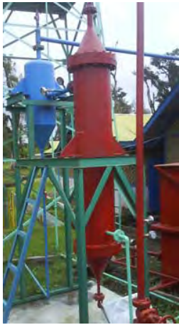
(a) Steam Generator
