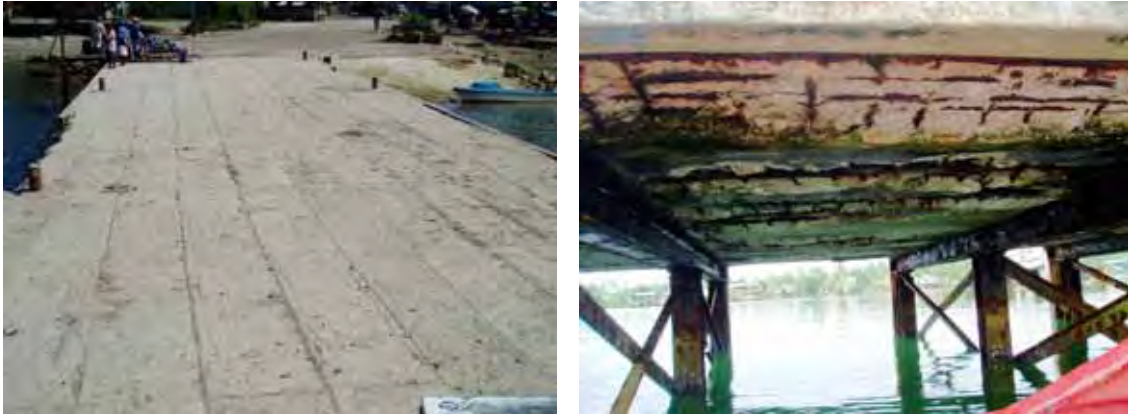
Photograph 1 State of deterioration of the existing jetty
