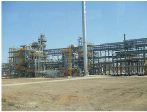
Oil refinery (sulphur recovery unit)
