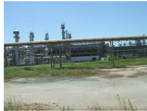
Gas refinery (sweetening unit)
