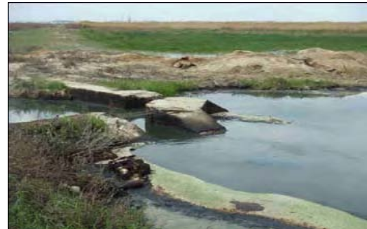
Waste water outlet in evaporation pond
