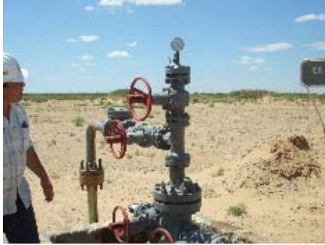
Injection of process water to underground
