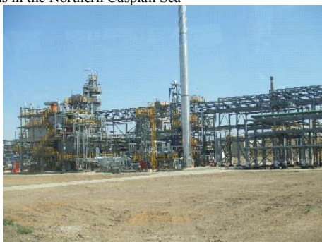
Desulfurizing facility in Atyrau oil refinery
