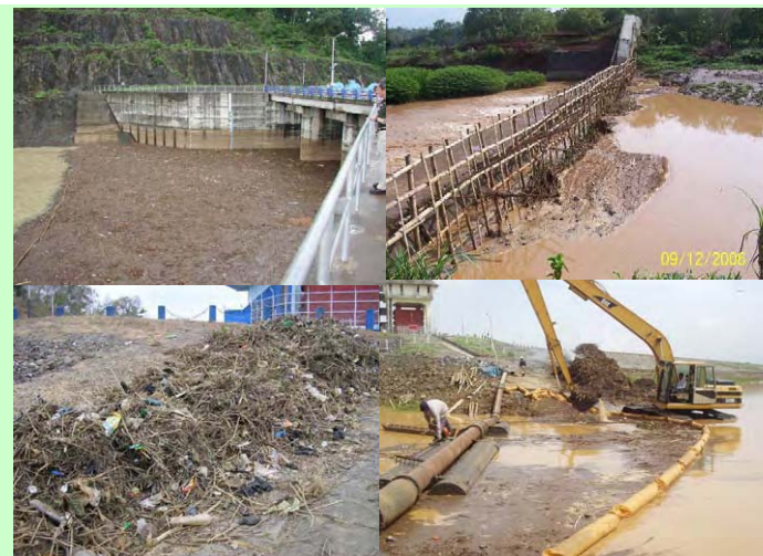
Garbage Problems at Intake
