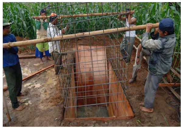
Construction of water tank (framework made of iron bar) at Slogohimo site
