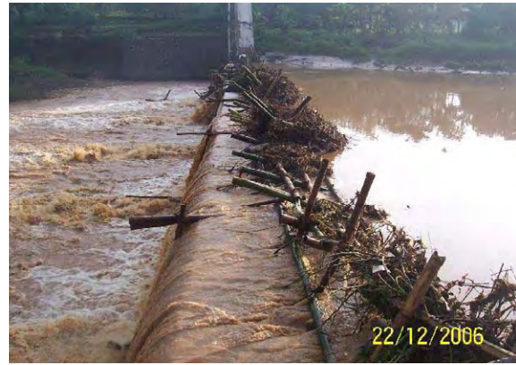
Garbage trap structure was broken by water pressure of big flood on December 22, 2006
