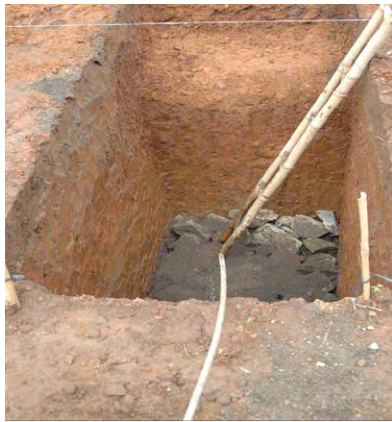
Construction of water tank at Slogohimo site (soil digging and rock foundation of lower portion of tank), tank capacity is 4 m 3 (2 m x 2 m x 1m)
