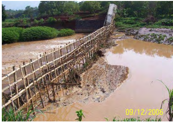
Garbage trap structure constructed in Keduang River. The trap successfully stopped the flow of the garbage on December 9, 2006
