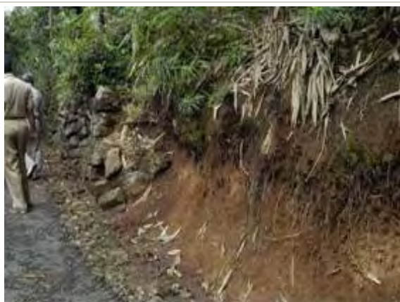
Road side erosion at settlement area in Wuryantoro watershed
