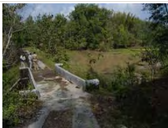
Check dam completely filled with sedimentation Constructed by IBRD project in Kamplong, Keduang watershed
