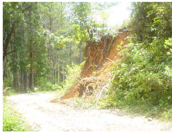
Road side erosion along village roads in Upper Solo watershed
