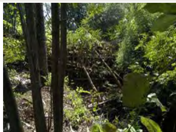
Urgent repairing of broken gully plug conducted by a community in Kerjo Lor, Keduang watershed
