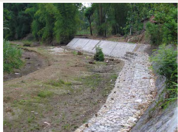
River bank protection in Tirtomoyo River
