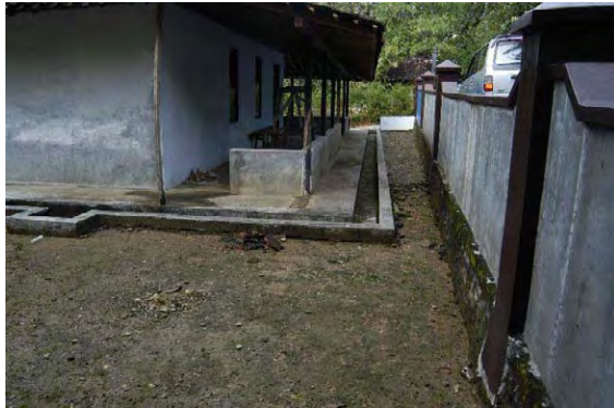
Side ditch collecting rain from roof constructed by IBRD project in Keduang watershed
