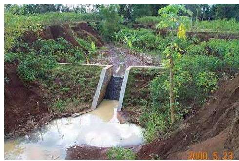
Large Gully Plug in Keduang Area
