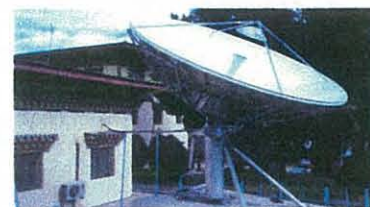
BBS Satellite Earth Station at Chubachu, Thimphu
