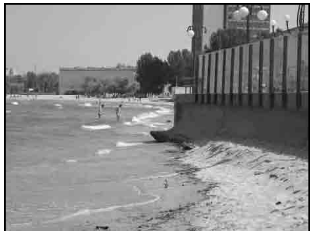
Photo-11 Toe Scouring of Beach Service Facility in Mamaia South
