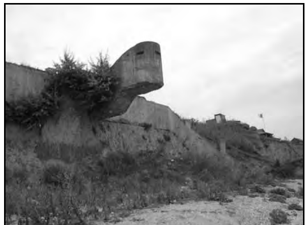
Photo-48 Cliff Scouring Condition in Schitu
