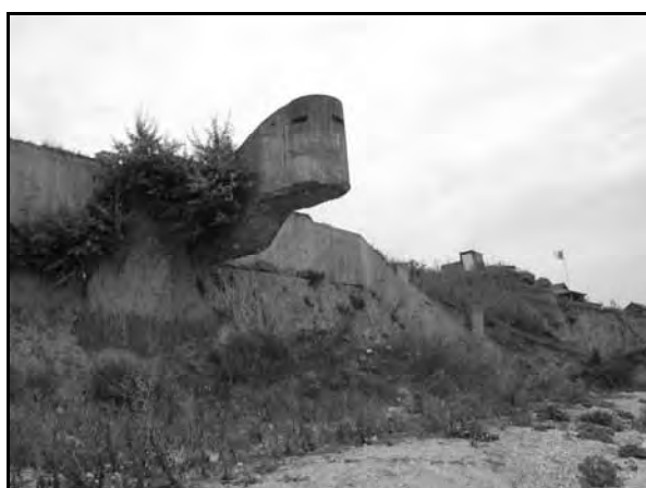
Photo-48 Cliff Scouring Condition in Schitu
