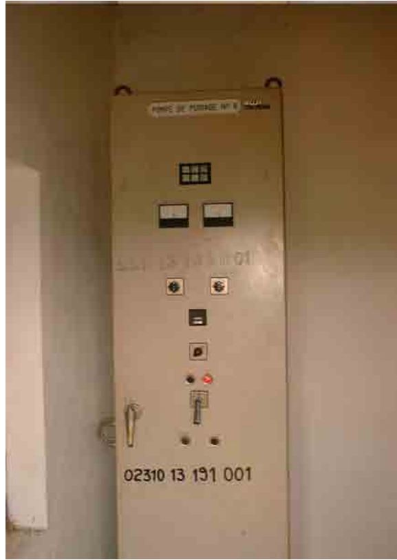
Well No.6: Operating Control panel
