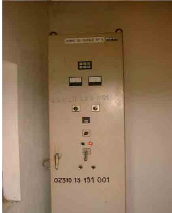
Well No.8: Operating Control panel
