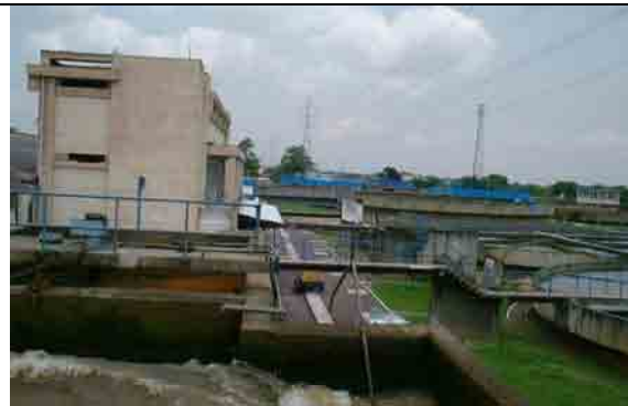
Existing facilities (Coagulation, Operation Building, Sedimentation) Under rehabilitation with the assistance of WB (Mod.1&2)
