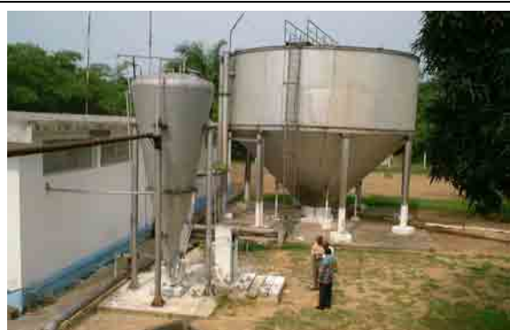
Compact Unit maid in DRC Coagulation and Sedimentation
