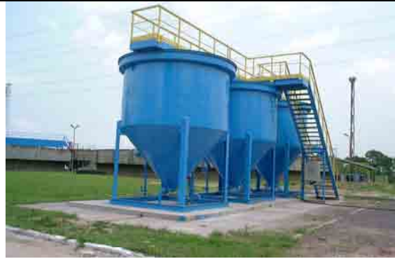
Mixing Tank for chemicals
