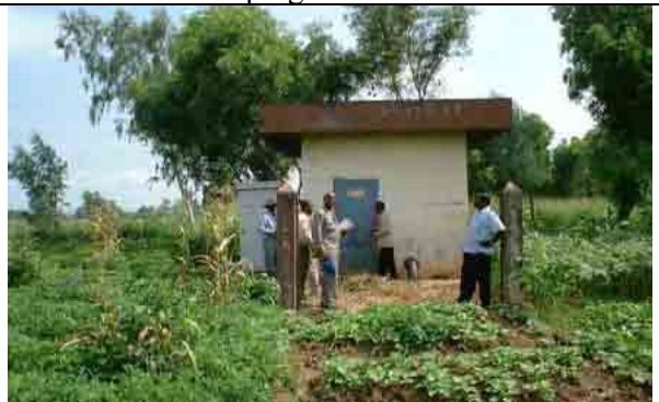
Well No. 3: Collapsed in 2004
