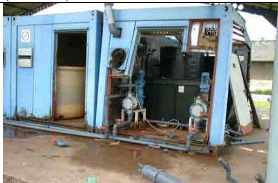
Chlorine Dosing Pump
