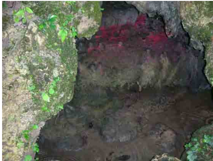
Plate 19: Leakage through the cavern near proposed dam axis on the left bank of the Seti River
