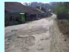
Poor Physical Accessibility in Kabupaten Majalengka
