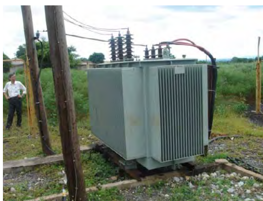
(Moatize 変電所:33/6.6kV 変圧器)
