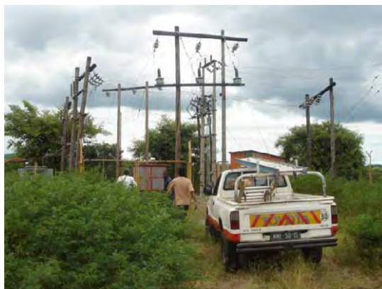
(Moatize 変電所:全景)
