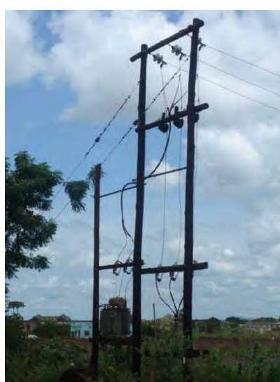
(Moatize 変電所:33kV 受電側)
