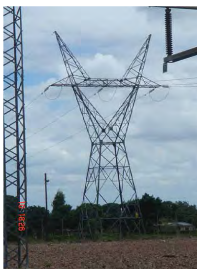
(Infulune 変電所:110kV 送電線)
