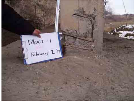
Damaged at the bottom of pier
