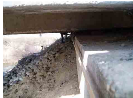
Deformation of the Abutment
