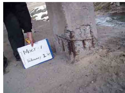
Exposure and Rusting of Re-bar (Pier)
