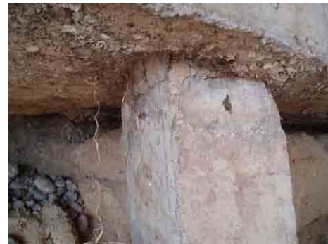
Damaged at concrete member of the bottom
