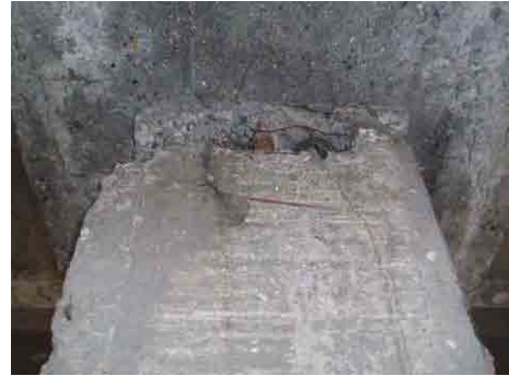
Damaged at the top of pier
