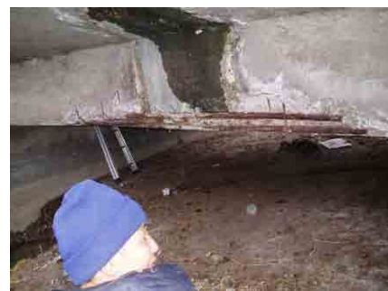
Exposure and Rusting of Re-bar (Girder)
