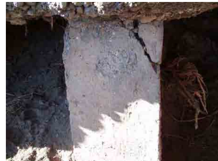
Crack of Pile Top
