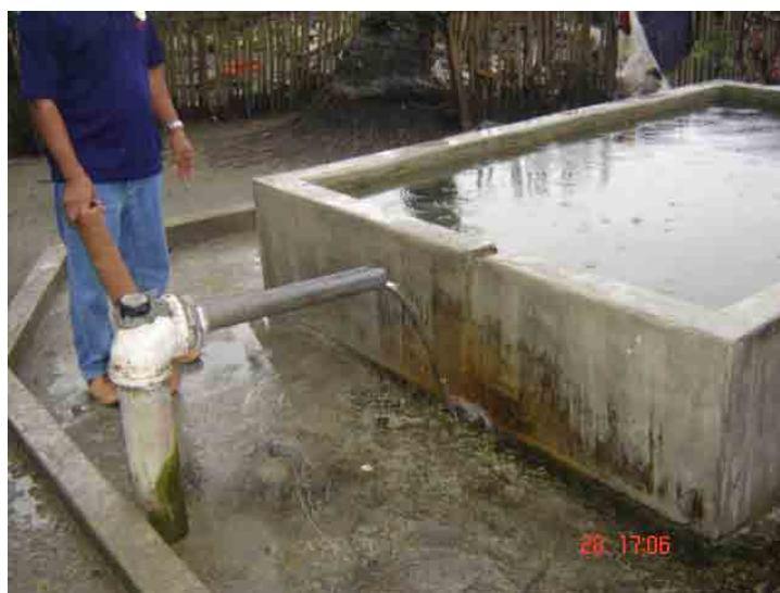
Figure 1. The free flowing water of the Level I facility
