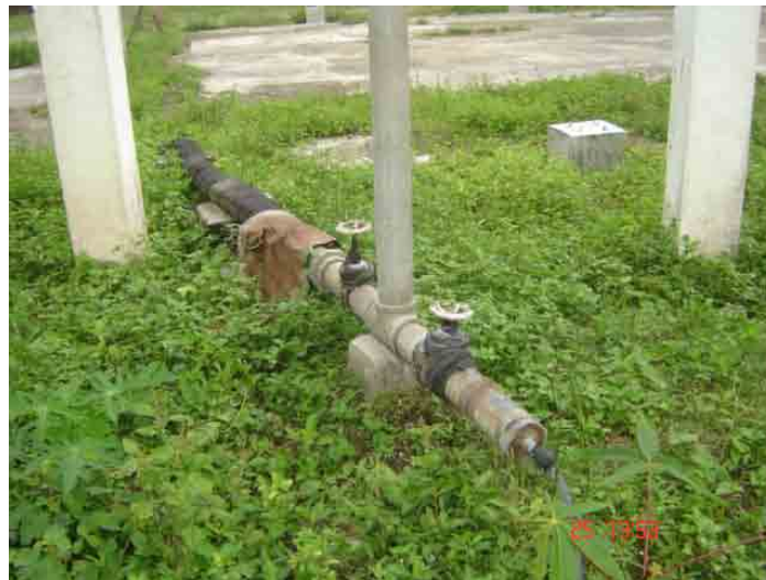
Figure 9. The discharge pipe from the reservoir
