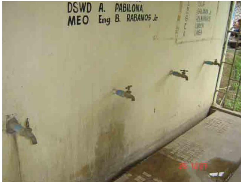
Figure 3. Faucets to distribute water to all members of LMaGWAS with steel fence.
