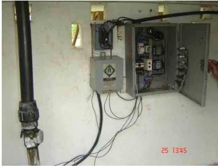
Figure 7. The control panel that controls the operation of the submersible pump and motor
