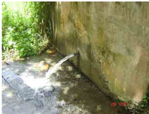
Figure 1. The spring box of the second source of water for Barangay Mayo Water System.
