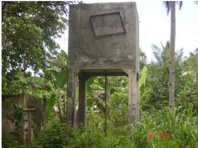
Figure 1. The reservoir of Maitum Guangguang Water System.
