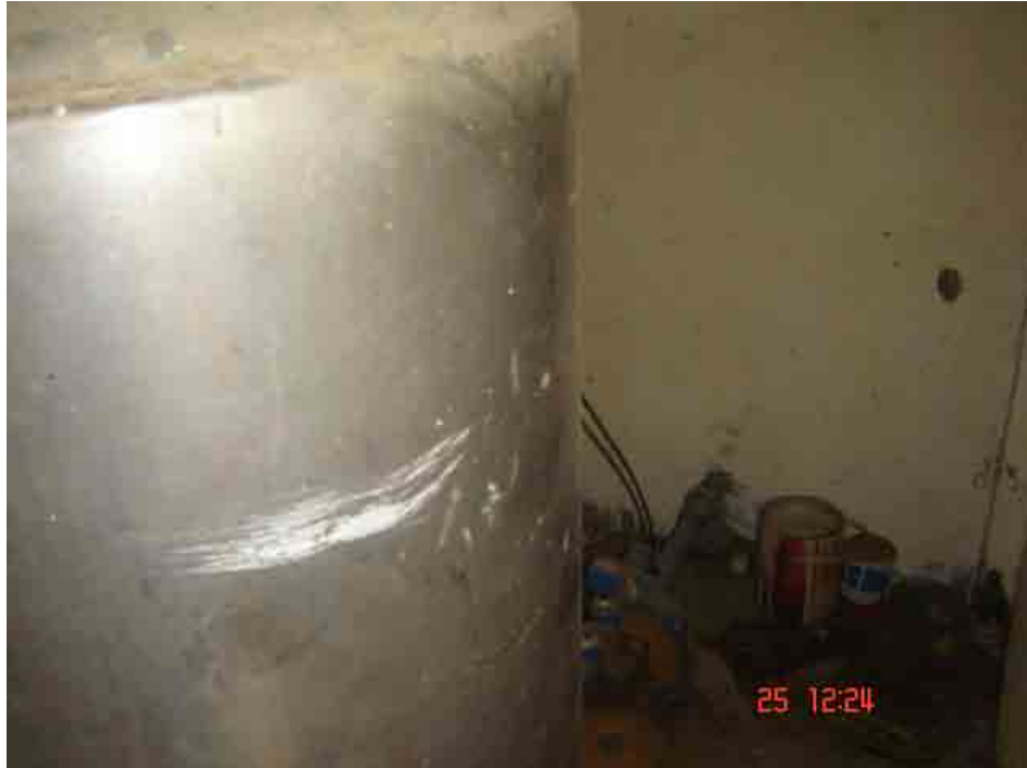
Figure 2. The pressurized tank located inside the pump house of LMaGWAS.
