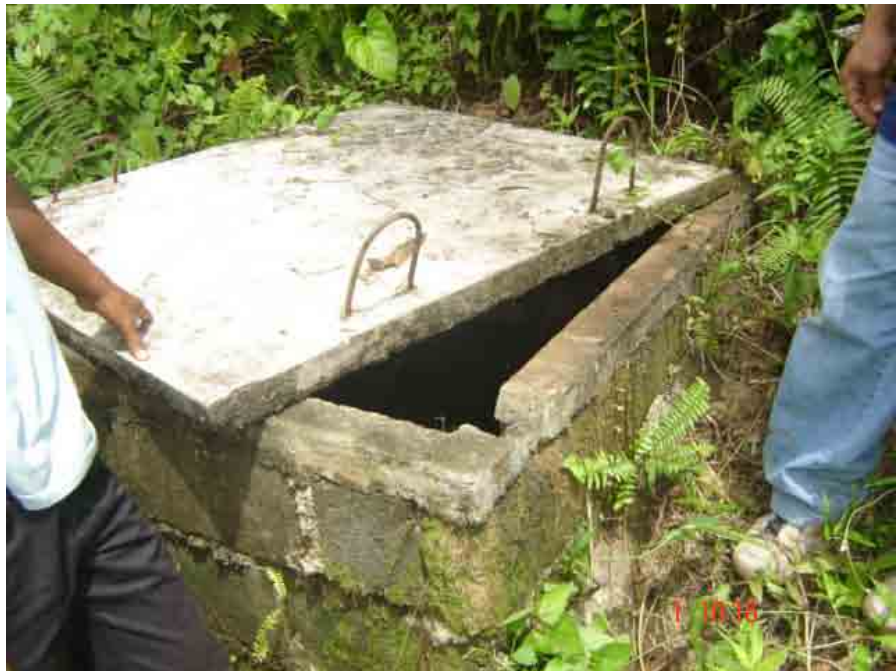
Figure 1. The spring inbox lined with hollow blocks as source of Olaycon Water System (Level I).
