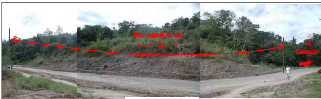
Photo 6.3 Front View of Damaged Section (Lagawe-Banaue Road Km 301)
