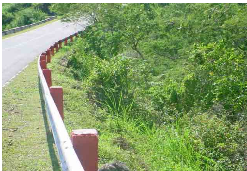
Figure 5.29 General View of Example DIS Slope for Road Slip
