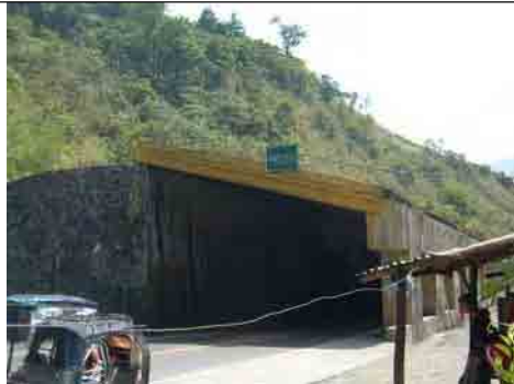
Rock shed to protect against rock slope collapse
