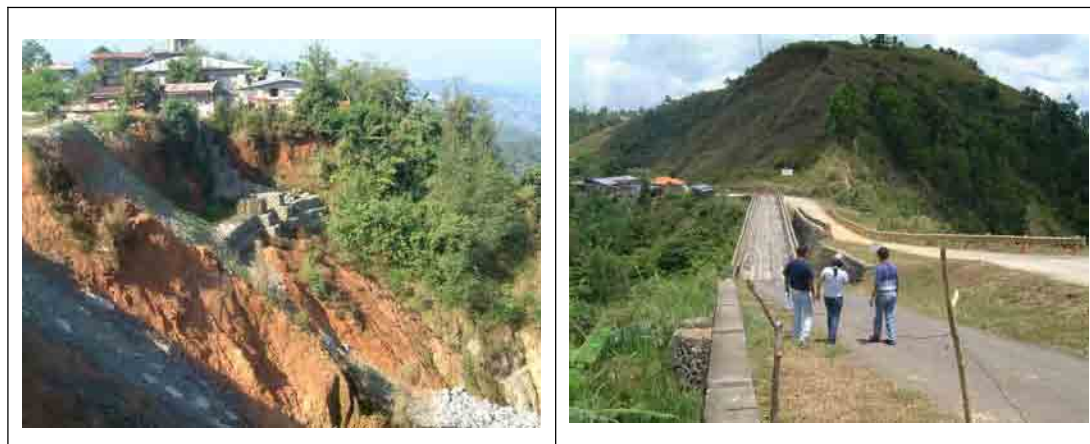
Figure 2.6 Road Slips Occurring on the Saddle Portion due to Erosion by Surface Runoff
