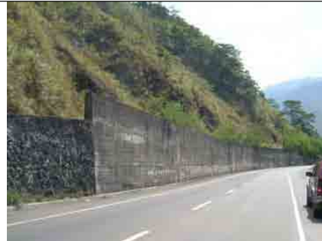
Concrete catch wall to protect against rock slope collapse
