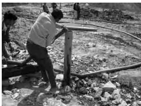
Photo 3.10 Check of Clogging in Pipe
