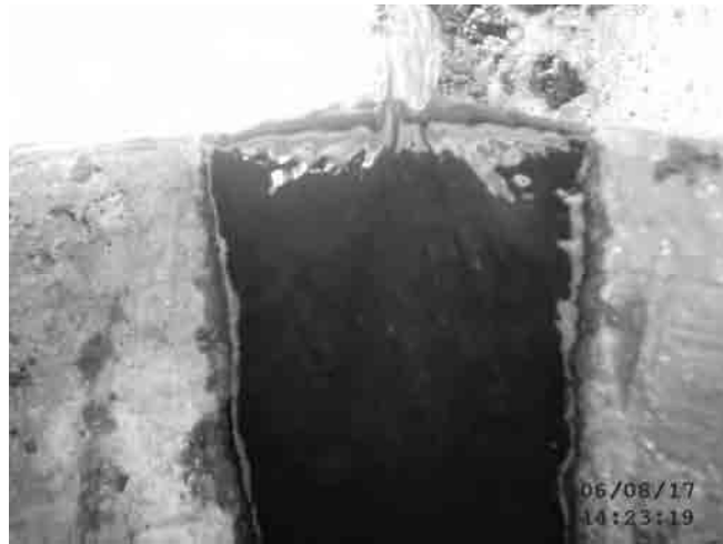
Photo 1 Leachate at the Exit of Main Collection Pipe before Tracer Test
