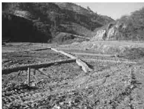
Photo 3.1 New Gas Ventilation Facility
