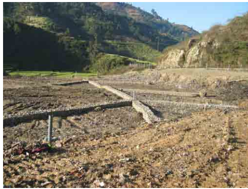
New Gas Ventilation Facility
