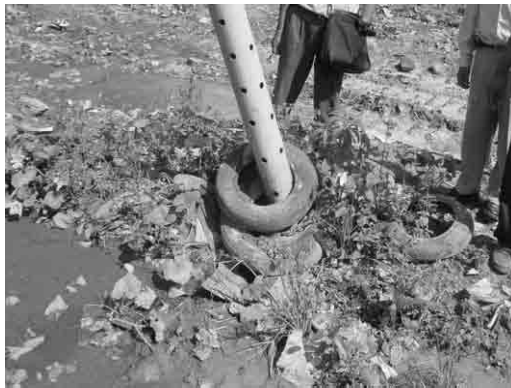
Gas Ventilation Facility with Used Tire
