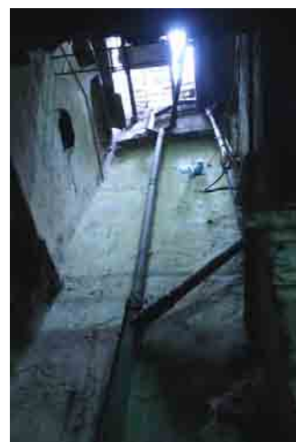
Exposed drainage in the common space
