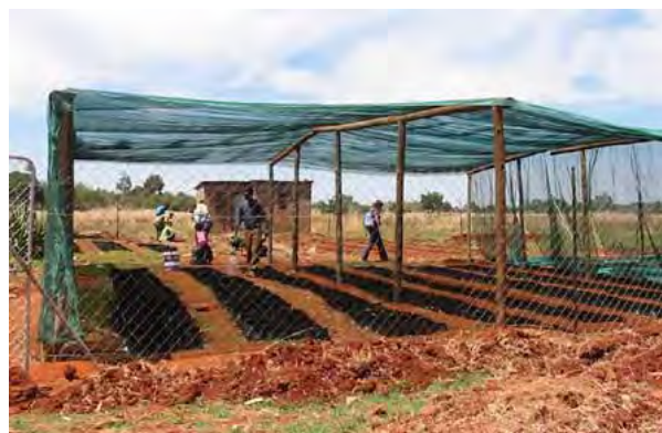
Photo 7-3-1 Nursery: Firstly, fences were installed to prevent livestock from entering the nursery. Secondly, pillars were put up and the seedlings were covered with a shading net in order to alleviate excessive sunlight. Then, beds with a depth of about 10 cm were dug and pots made from plastic bags were put in to it in order to grow the seedlings. (Ga-Kopane village)
