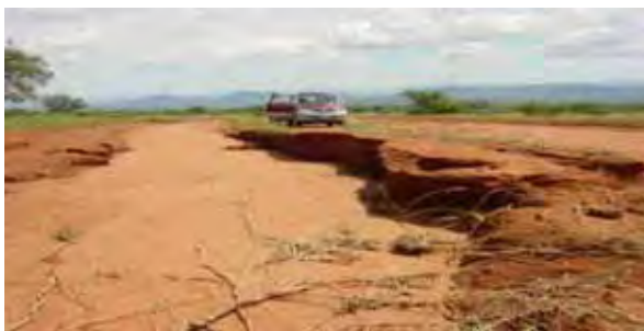
Photo 7.6-5 Damage caused by a flood occurred on 3rd March 2006 in Mankotsana
