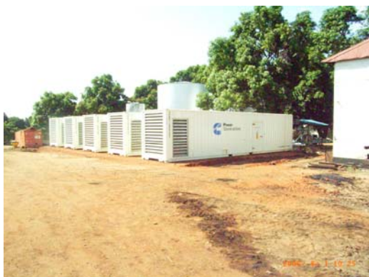
New Generators (1MWx5)
