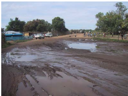
Unpaved Road Condition after Rain
