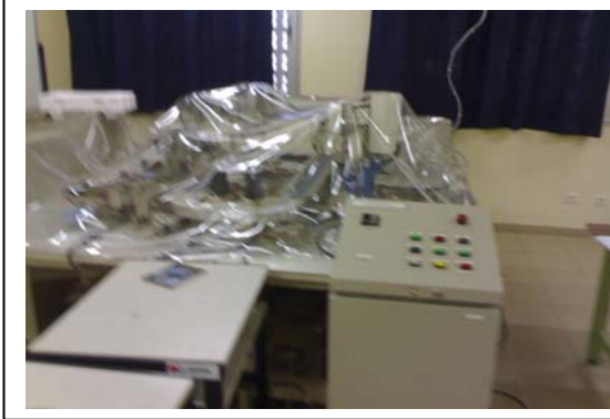
Automatics: Control equipment
