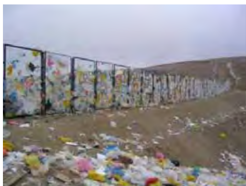
<Embankment Dam and Litter Control Fence> Embankment Dam was constructed on the south edge of the landfill area and litter control fence was installed on the dam.
