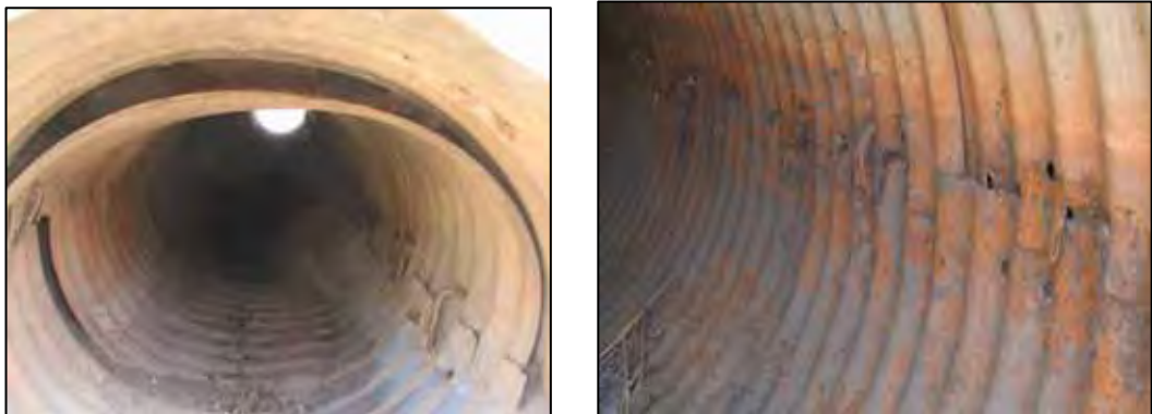
Photo 2.2 State of Damage in Corrugated Metal Pipe Culverts
