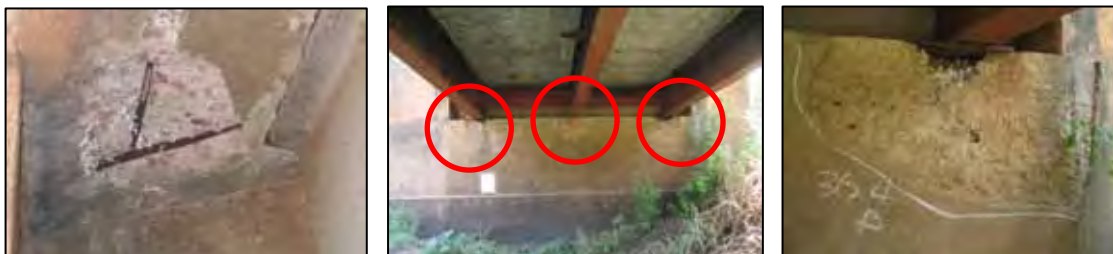
Damage to floor plate concrete
