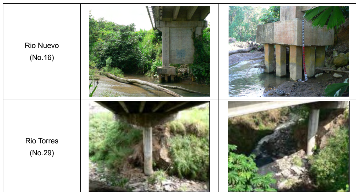
Figure11.7.4. Scouring of Riverbed around Pier
