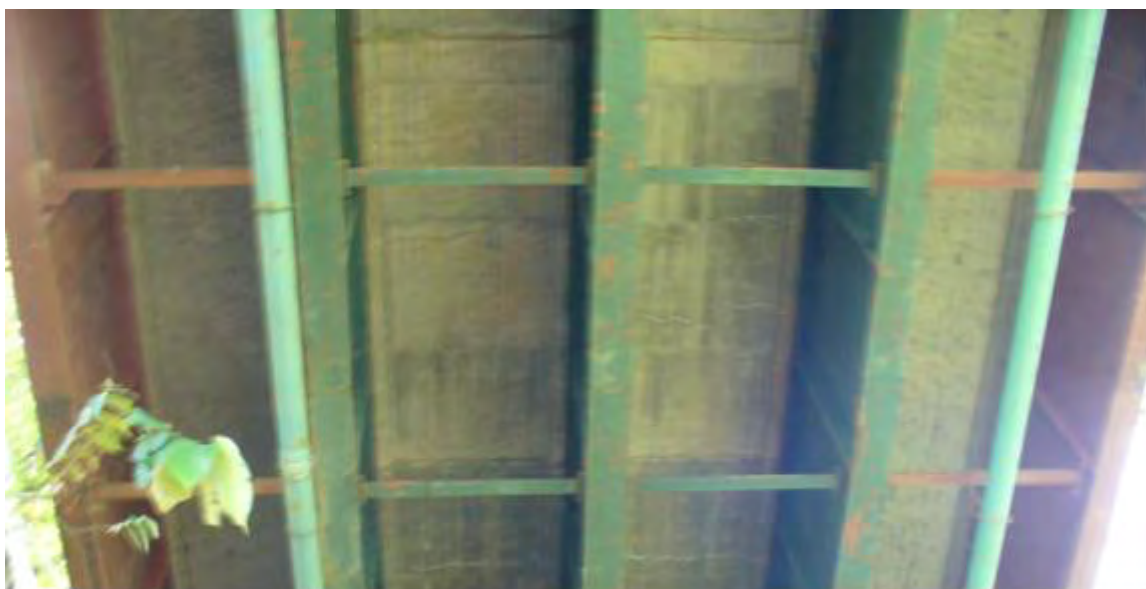
Figure 11.1.3. Crack on Deck Slab of No.19 Sarapiquí Bridge
