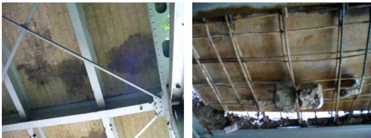
Figure 11.1.2. Damages on Deck Slab of Truss Bridge
