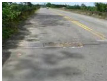
(a) Broken Expansion Joint
