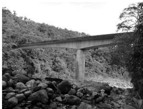
Figure 10.3.4. Large Rock Deposit on No.20 Sucio River Bridge
