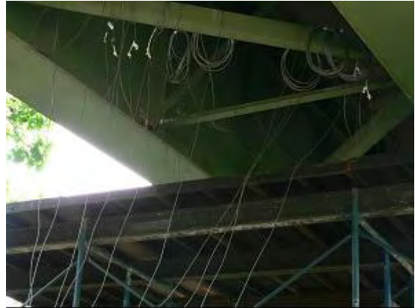
Gauge Cable Connection
