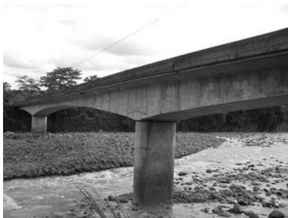
Figure 10.3.3. Large Rock Deposit on No.17 Chirripo River Bridge
