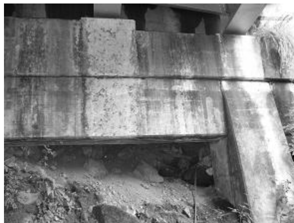
Figure 10.3.2. Erosion of Backfill on No.12 Puerto Nuevo Bridge
