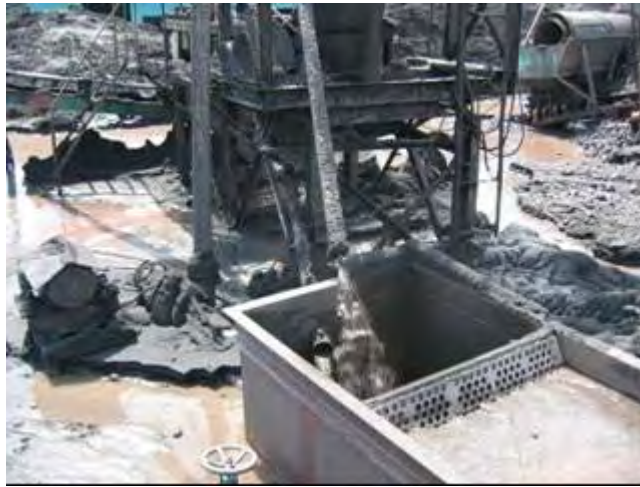
Photo 5-2-1 Overflow Bypass Pipe
