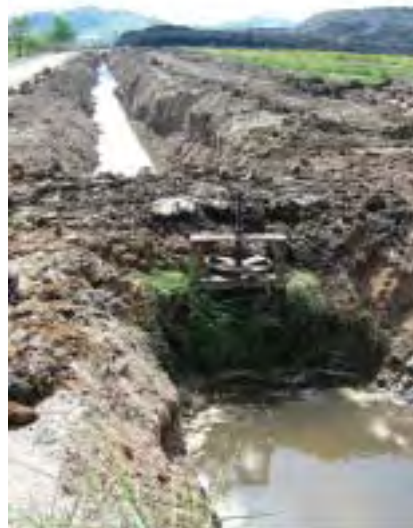
Photo 5-2-7 Water Channel for Recycling water
