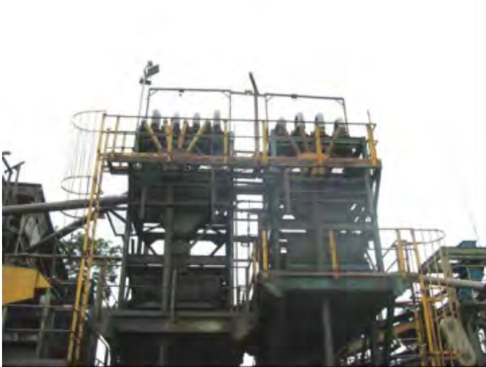
Photo 5-2-2 Eight cyclone classifier feed pipes
