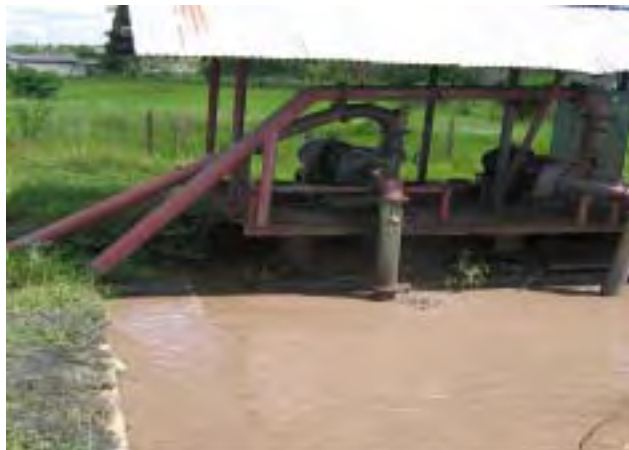
Photo 5-2-3 Facility Designed to Recycle Jigging Water
