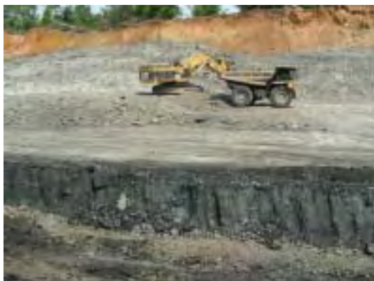
Photo 3. Dirty coal removed during work for cleaning of the upper coal layer
