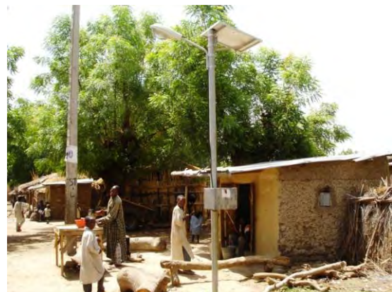
6) SL: The light is sodium light with an input of 18 W. The light turns on and off automatically and can be used for 6 hours a day (4 hours from sunset and 2 hours before sunrise). The PV module is as the same as for BCS (60 W), and the storage battery is as the same as for SHS (65 Ah).
