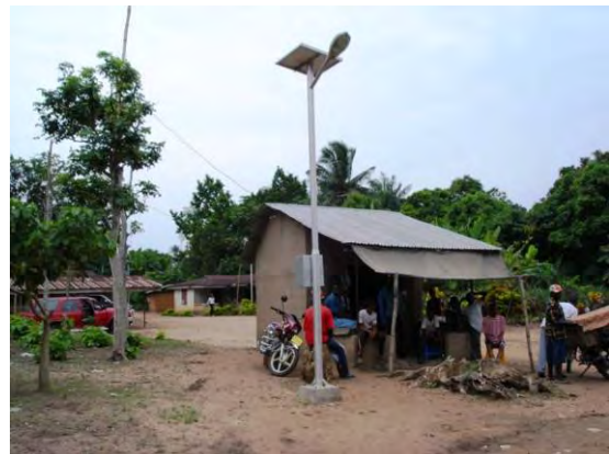
6) SL: The PV module is as the same as for PF (62 W), and the storage battery is as the same as for SHS (60 Ah). The lighting is a fluorescent light with a capacity of 20 W. The light turns on and off automatically and can be used for 4 hours a day (4 hours from sunset).
