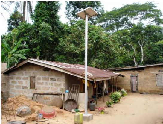
5) SHS: The PV module is as the same as for PF (62 W). Two (2) units of CFL and a DC outlet are installed inside. The storage battery is sealed type with a capacity of 60 Ah.
