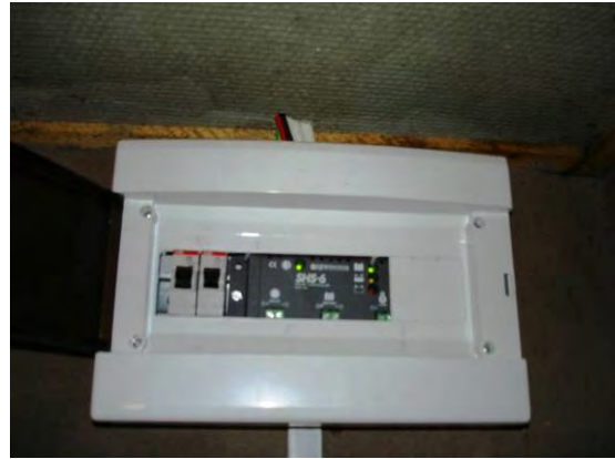
4) Junction Box for SHS: The box contains the charge controller (6 A) and Molded-Case Circuit Breaker (MCCB). The charge controller has indicators which show the voltage level of the storage battery.
