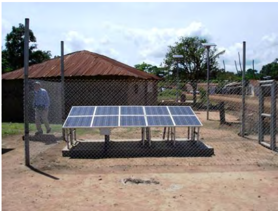
3) PV array for PF: The PV modules are the same as in Jigawa (60 W), and ten (10) units of module are installed. Six (6) of them are used for lighting, and four (4) of them are used for a PV vaccine refrigerator.
