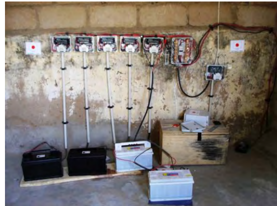
2) BCS Station (internal): The number of charging circuits is five (5) with a rated current of 20 A. The storage batteries are vented-type with a capacity of 88Ah.
