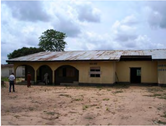
1) PF (meeting hall): Twelve (12) units of 11 W Compact fluorescent lamps (CFLs) are installed inside.
