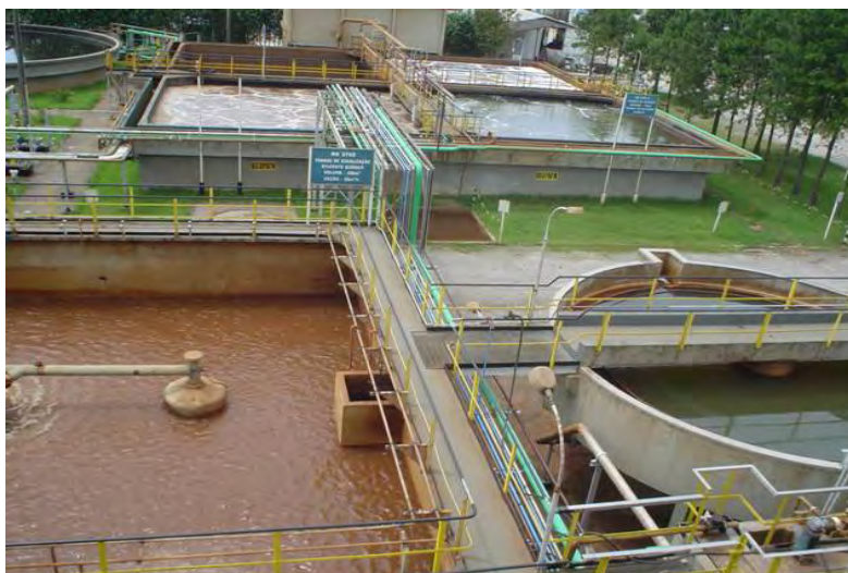
Photo 6.4.3 Solvay Indupa Facility operation status
