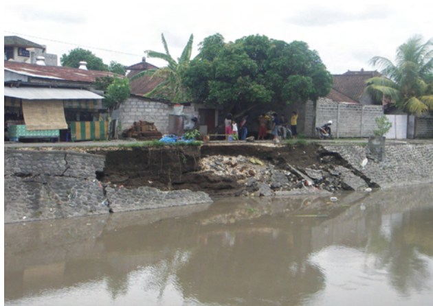
Figure-III-4.1 Photos of Damage Condition by Flood December 12, 2005
