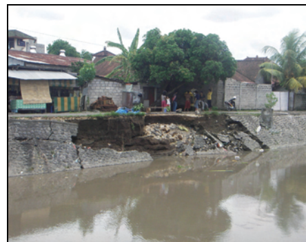
Bank Slope Failure near Upstream of JL. P. Misol (From Left Bank Side)
