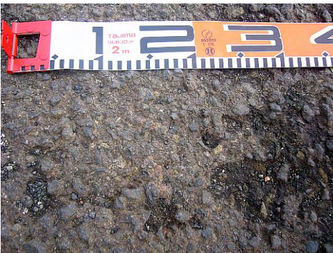
Section F-3 STA. 13+300 Ravelling nearby Airport
