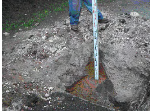
Roadbed soil exposed at opposite side
