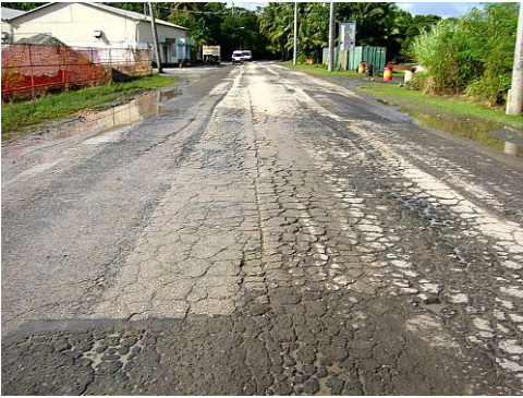
Section F-1 STA. 9+800 Flood Section, Alligator Cracks and Ravelling
