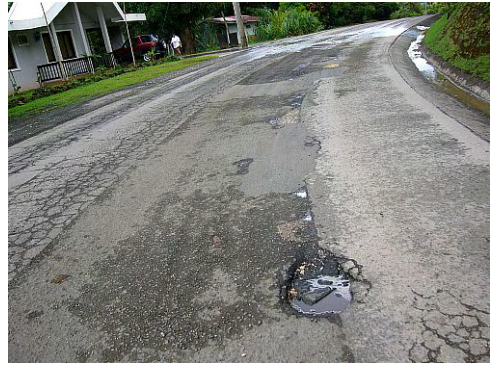
Section F-1 STA. 10+350 Alligator Cracks and Ravelling
