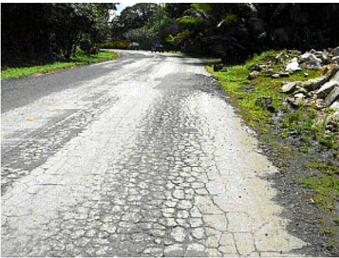
Section F-1 STA. 12+400 Alligator Cracks and Ravelling
