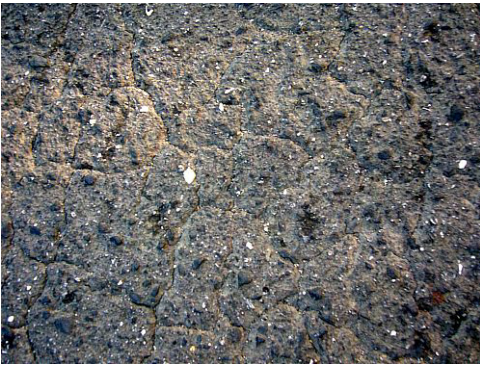
Section C STA. 6+860 Ravelling and Cracks where Shell remains
