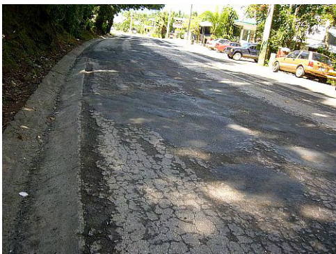
Section C STA. 5+800 Alligator Cracks
