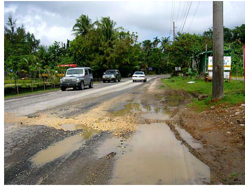
Section B STA. 2+450 Alligator Cracks, Drainage Problem
