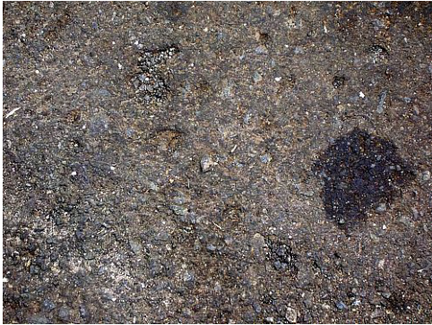
Pavement damage at the parking lot without roof
