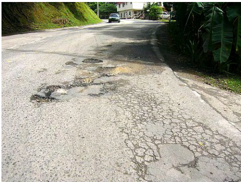
Section B STA. 2+450 Alligator Cracks and Ravelling
