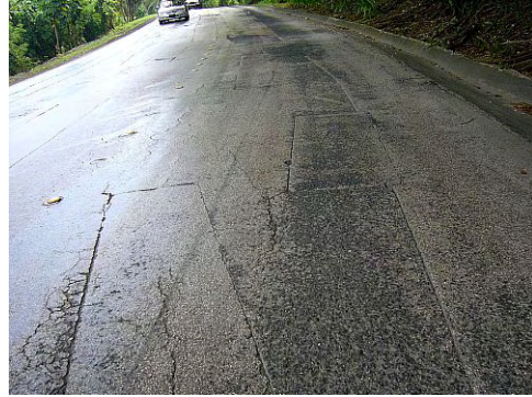
Section E-1 STA. 1+500 Ravelling
