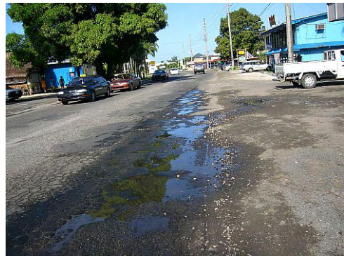
Section A STA. 4+080 Alligator Cracks, Grooving/Rutting and Ravelling
