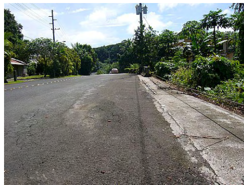
Section C STA. 6+000 Ravelling at Land-slide
