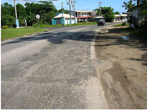
Section E-1 STA. 1+100 Alligator Cracks and Ravelling
