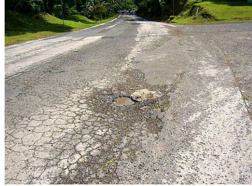
Section C STA. 6+150 Alligator Cracks and Ravelling
