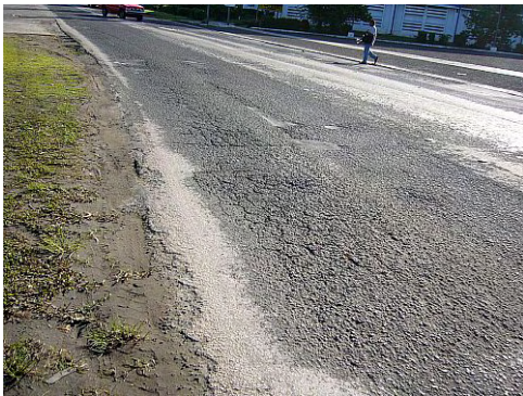
Section A STA. 3+720 Alligator Cracks, Grooving/Rutting and Ravelling
