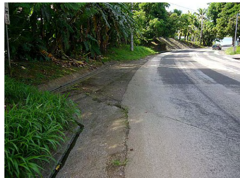
Section D STA. 0+280 Alligator Cracks
