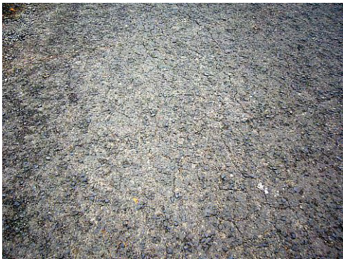
Section E-2 STA. 3+180 Cracks and Ravelling
