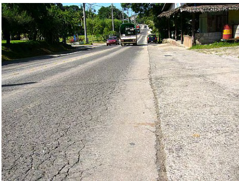
Section A STA. 5+300 Alligator Cracks, Grooving/Rutting and Ravelling
