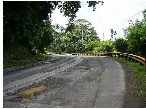
Section C STA. 7+320 Alligator Cracks and Ravelling
