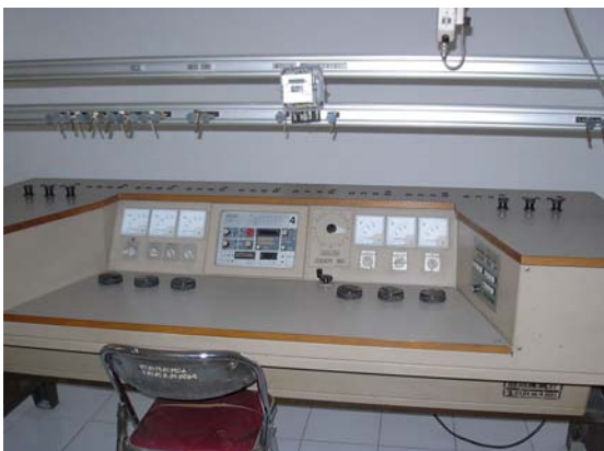
Photo 5.7.3.2 Test stand for kWh meter (Surabaya)
