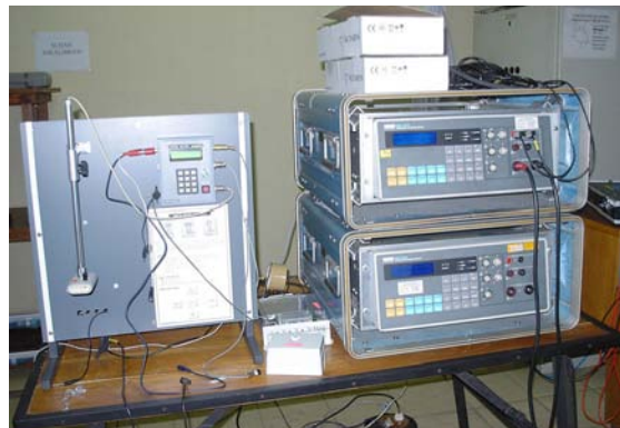
Photo 5.7.2.4 Reference standard meter for kWh
