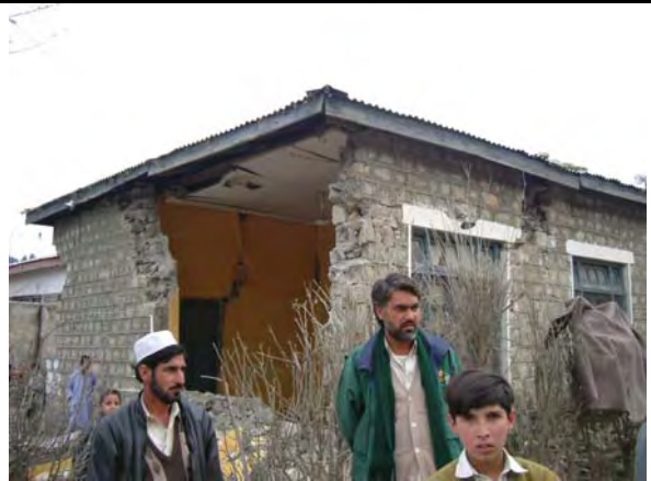
Wall damaged (Staff House)
