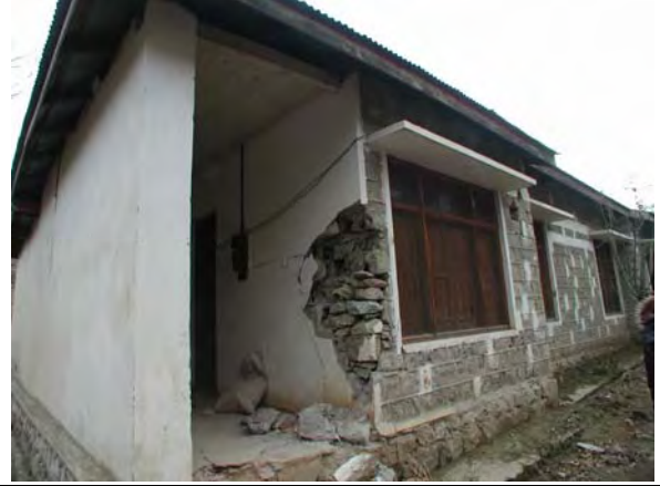
A part of wall damaged (Staff House)
