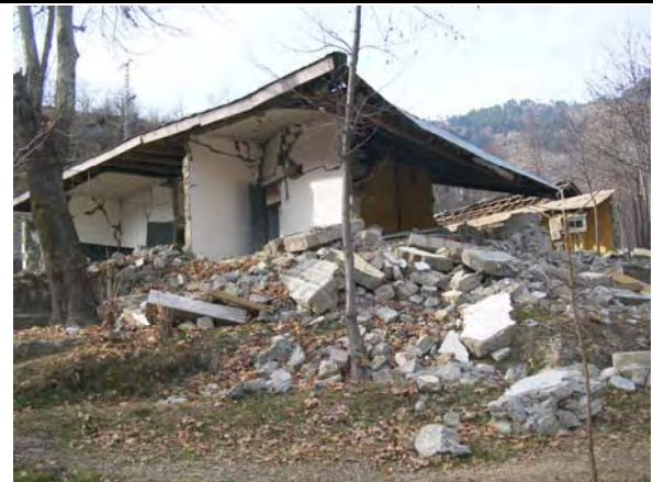
Collapsed staff house
