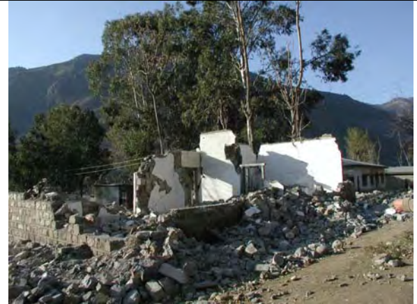
Collapsed Guard House
