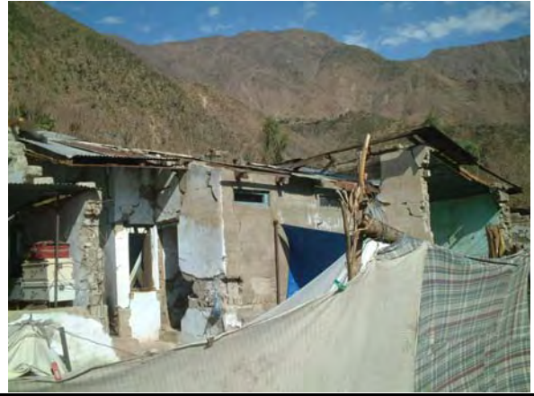
Collapsed staff house
