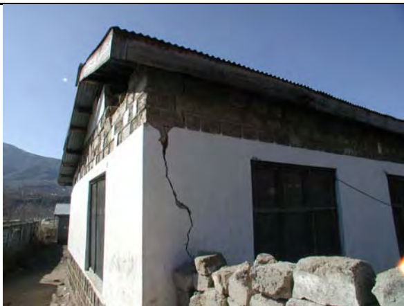
Wall greatly damaged (OPD)
