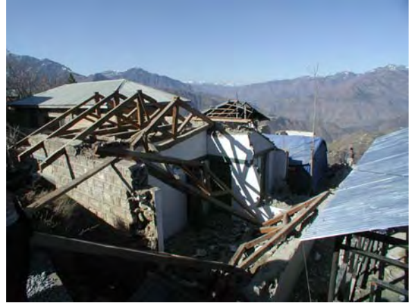
Greatly damaged staff house
