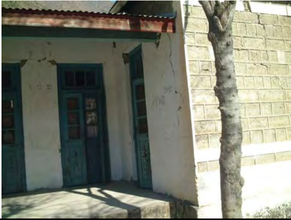
Greatly damaged OPD
