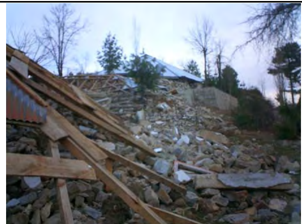
Collapsed staff house
