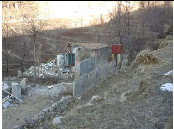
Collapsed staff house
