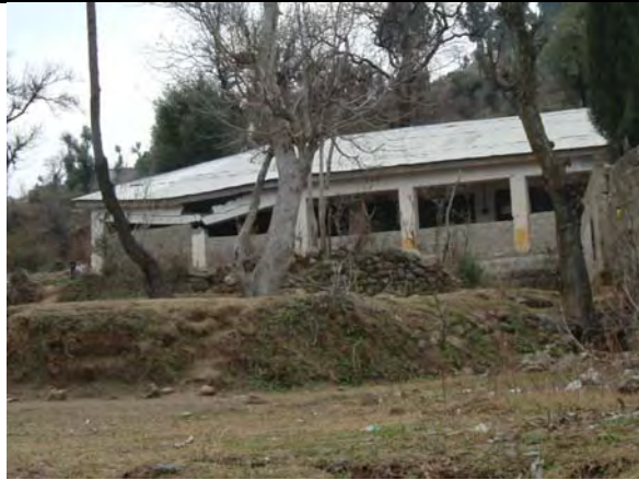
Greatly damaged OPD
