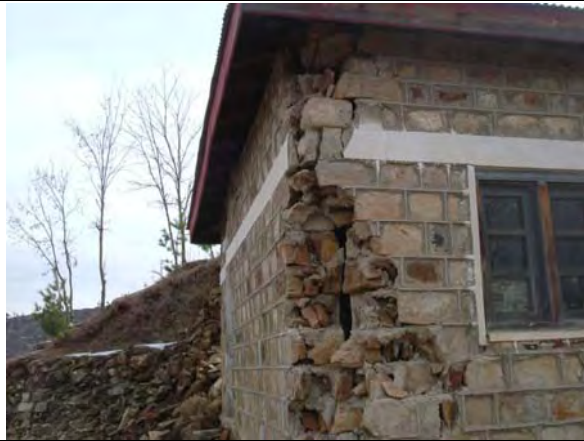
A partly damaged OPD
