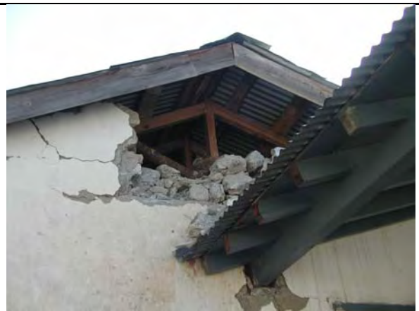
Collapsed staff house
