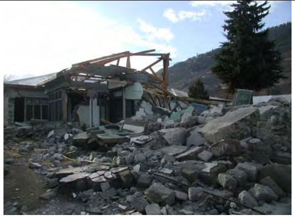
Collapsed staff house
