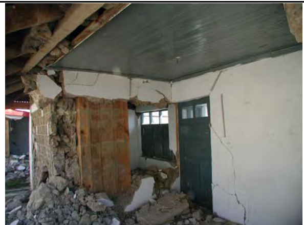
Greatly damaged staff House
