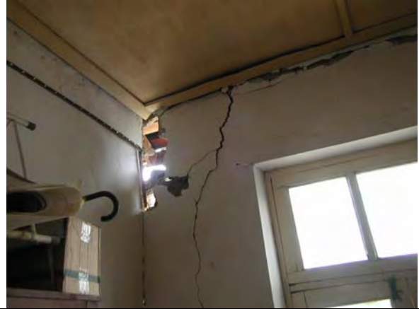
Greatly damaged OPD
