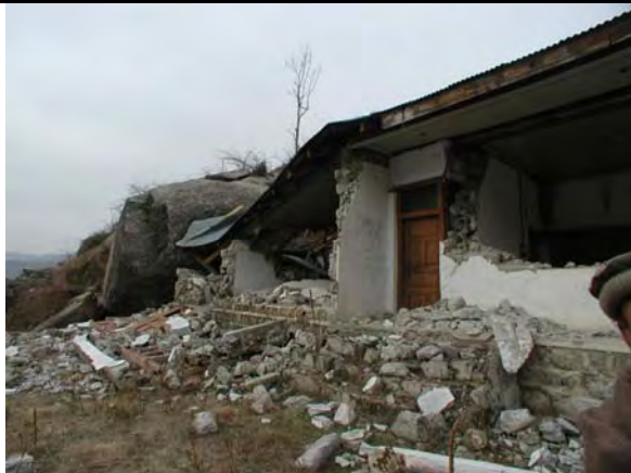
Collapsed Doctor's House
