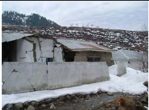
Collapsed staff house
