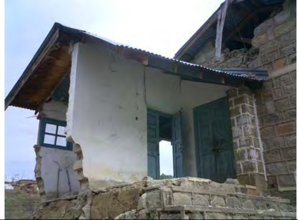
Collapsed staff house
