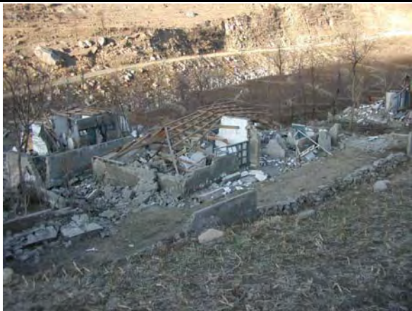
Collapsed OPD and Wards
