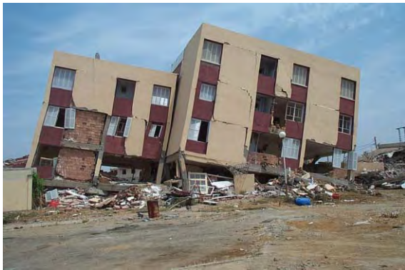
c) Destruction by Column Collapse
