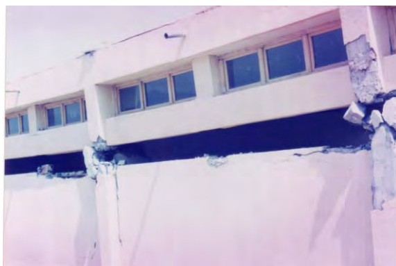
a) Shear Failure of Short Column
