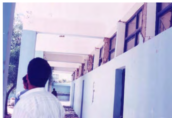
b) Flexural/Shear Failure of Column
