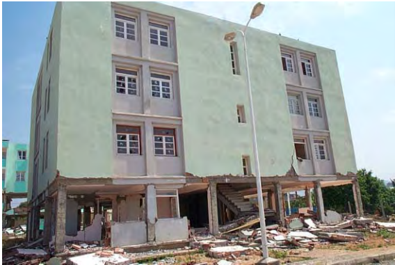
a) Heavy Non-structural Damage at 1 st storey
