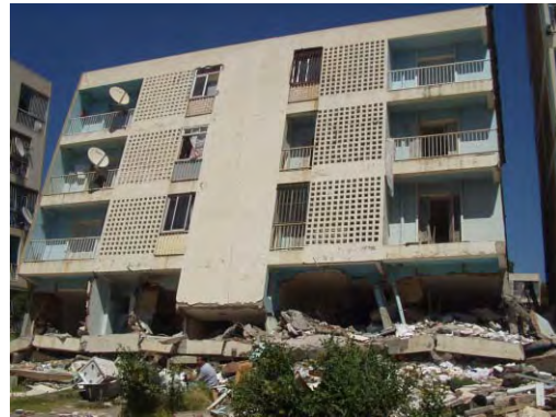
b) Destruction by Column Collapse
