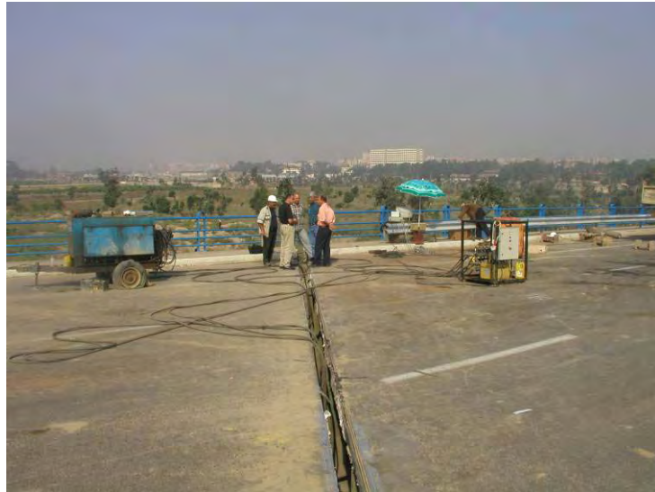
Figure 6-27 Displacement of a Girder of EL HARRACH Bridge
