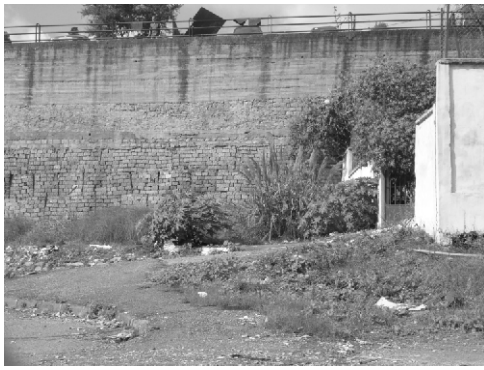
Photo 5-9 Wall Broken by Landslide
