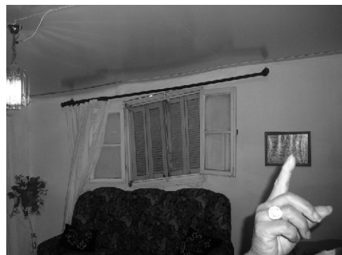
Photo 5-7 Window Broken by Landslide
