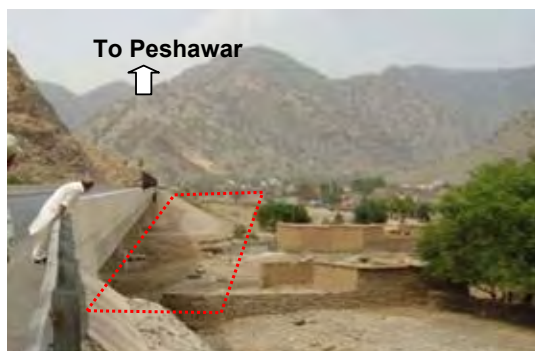
A Piece of Private Land located at No.6AR Bridge Construction Site (River Bed) at Sta.21+260
