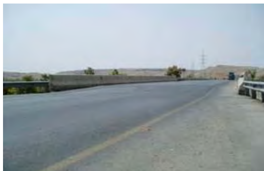
Settlement of Bridge Approach (Bridge No.3)
