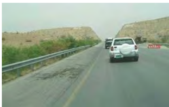
Damage of Shoulders
