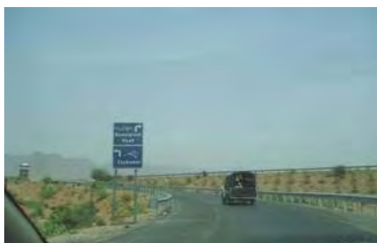
Kohat Link Road On-Ramp, No proper On-ramp for South
