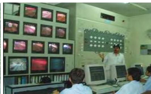
CCTV Monitoring and Control Board
