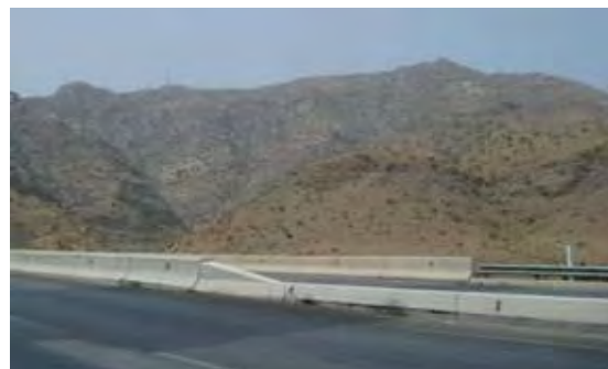
Settlement of Bridge Approach (Bridge No.4)
