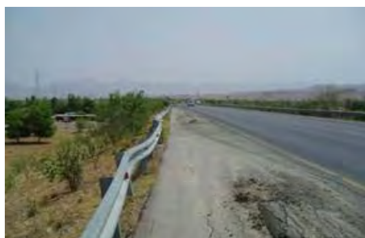
Shoulder / Guard Rail Damages
