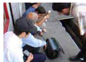
(Fig6 Leakage detection)
